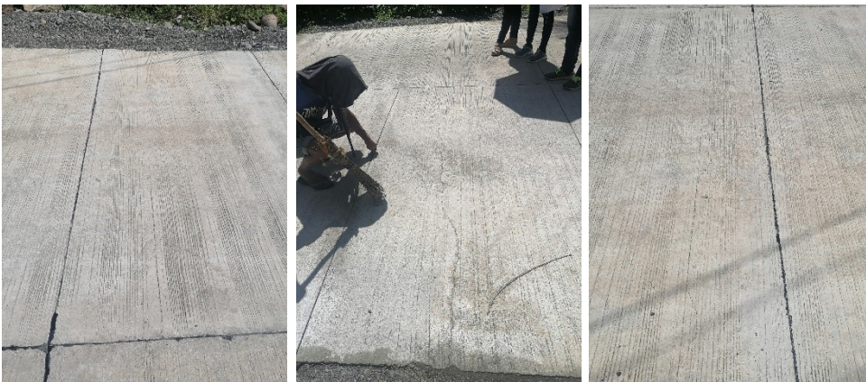
PCCP blocks with transverse cracking within 1.5 meters from weakened plane joints
