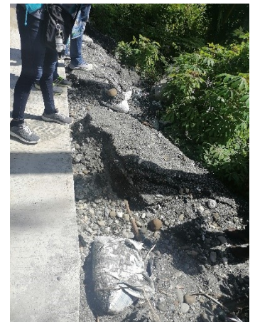
Uncompact or loose road shoulder
