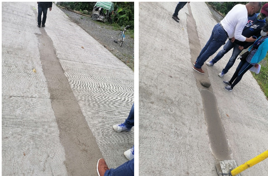
Quality of plastering of the affected PCCP blocks with water ponding under observation prior to the release of retention fee
