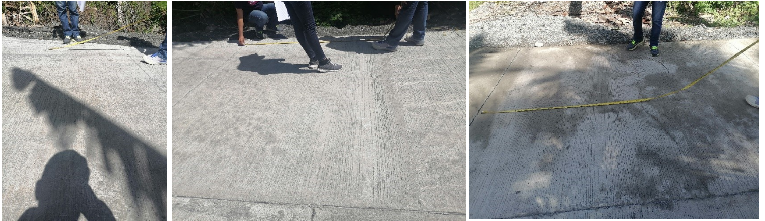
PCCP blocks with transverse cracking within middle block
