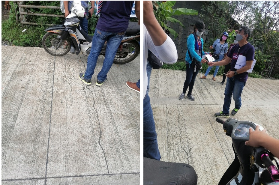
PCCP block with transverse cracking within 1.5 meters from weakened plane joints
